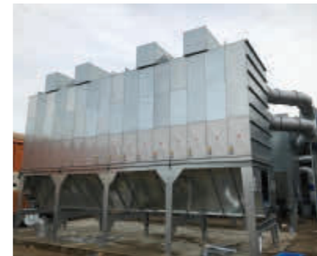
Air Plants installations in operation – dust cyclone, dust extraction system and fansets.
