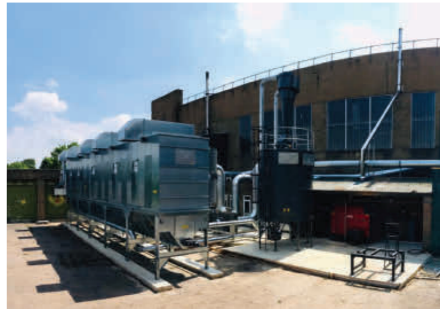
Air Plants Modulair dust extraction system working in tandem with a Talbott's silo and Talbott's Modern Wood Energy 199 biomass boiler.
